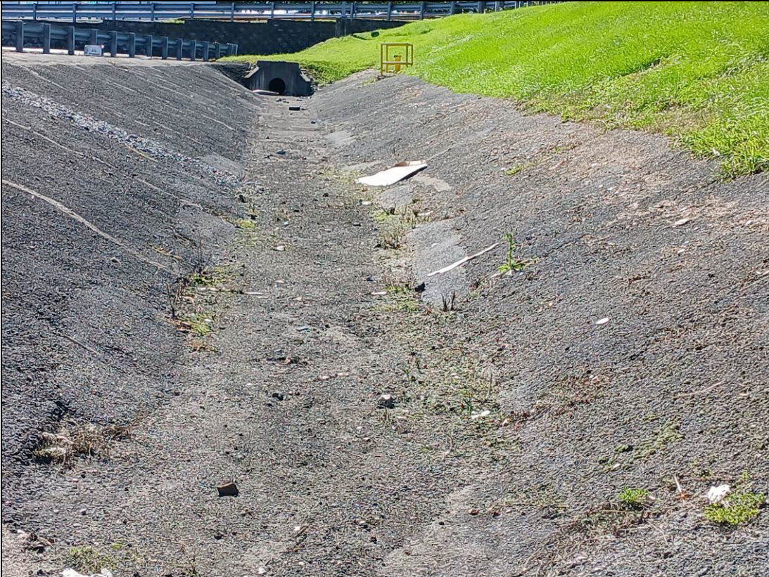
Photo 2: Photo looking south at vegetation growing the in paved swale. Trash was removed from the swale during the inspection.
