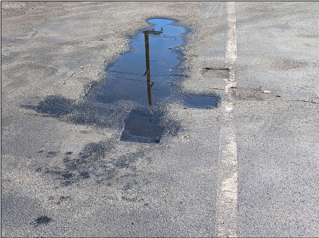
Photo 4: Photo looking east at impressions in the asphalt from the trailer feet. Cap is intact at impression locations.
