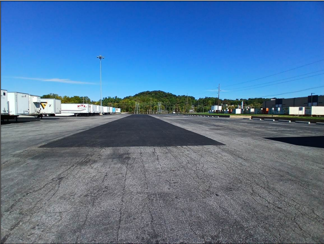
Photo 5: Photo looking north at area of asphalt repair in the central portion of the WPL.
