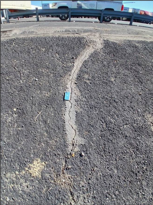
Photo 3: Photo looking east at a crack in eastern slope of the paved swale.
